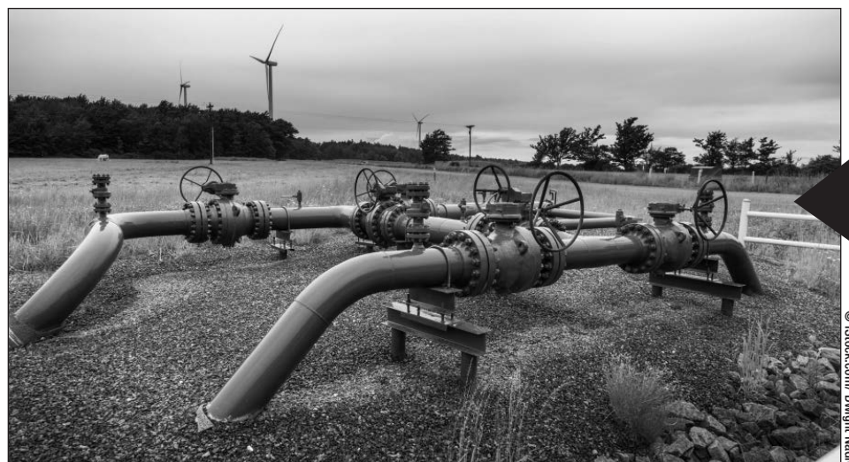
Shale gas pipelines in the USA
