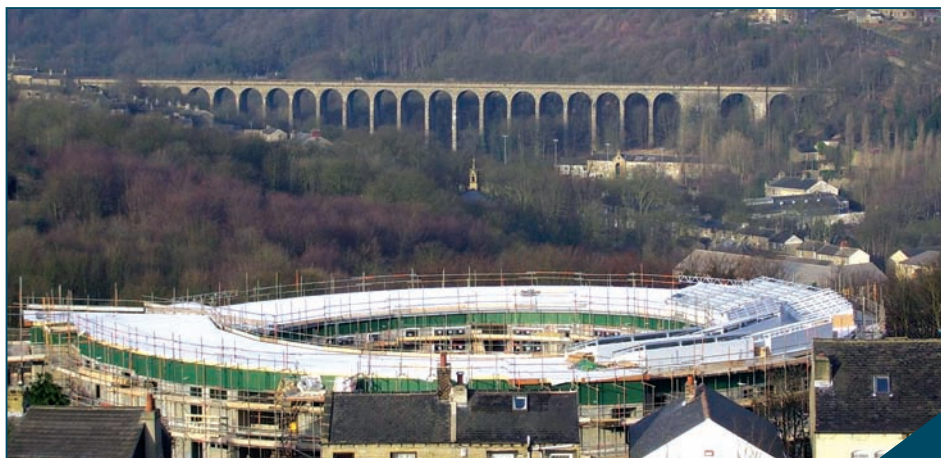
The 'Circus': a new social housing development in West Yorkshire incorporating solar panels
